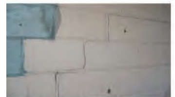
Cracks in block CA. manufacturing plant
