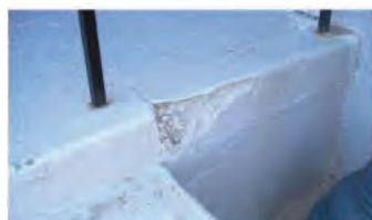
Spalled concrete CT. airport office
