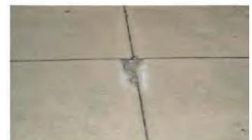
Broken concrete VA. parking garage
