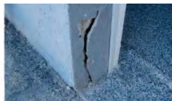
Cracked stucco FL. distribution center
