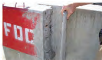
Broken concrete VA. parking garage
