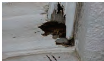
Rotted wood N.C. apartment complex
