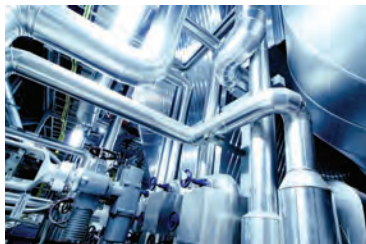
Typical high-corrosive environment — central utility plants.
