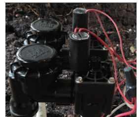
Ignition & Sprinkler Systems
