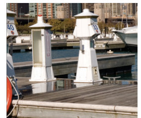
Marine Shore Power & Dock Lighting
