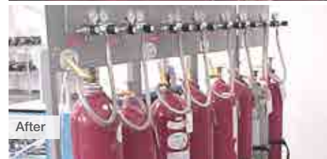
Photos courtesy of Praxair Specialty Gases
