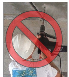
No overhead drilling!
